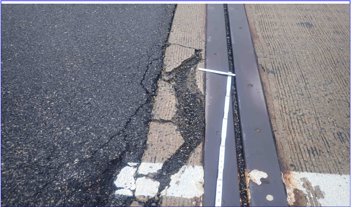
9. SPAN 3 STRIP SEAL JOINT HEADER LARGE SPALL IN THE LEFT LANE LOOK DOWN & S
