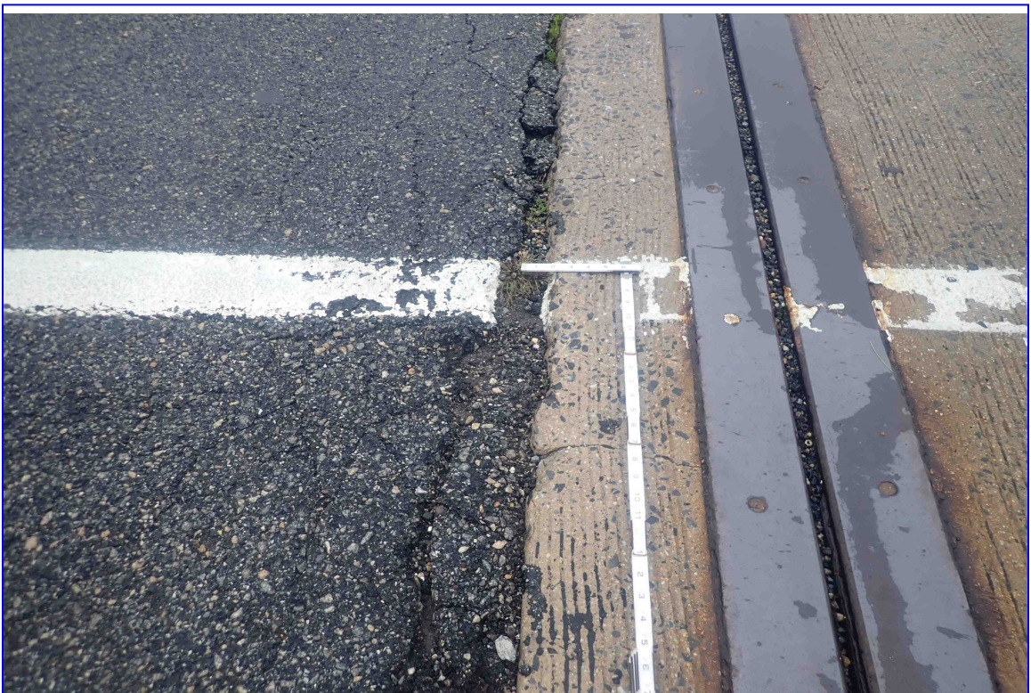
10. SPAN 3 E APPR SLAB LARGE DEEP SPALLS IN ASPHALT OVERLAY AT HEADER LOOK S
