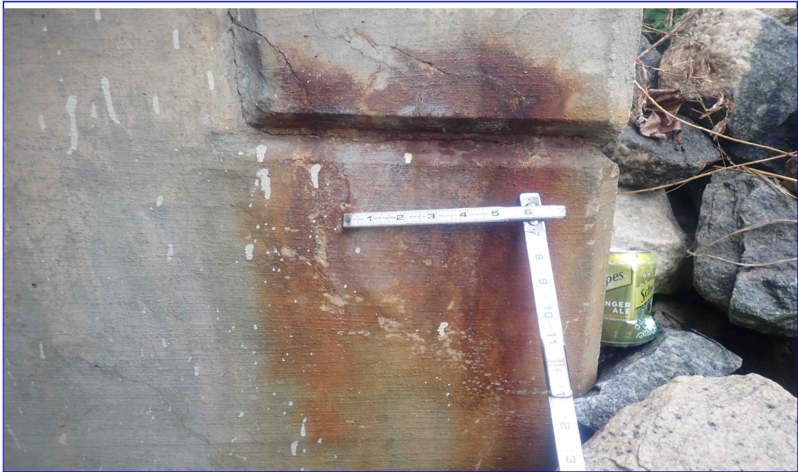
19. SPAN 1 WEST ABUTMENT BREASTWALL RUST STAIN & CRACK ON EAST FACE LOOK W
