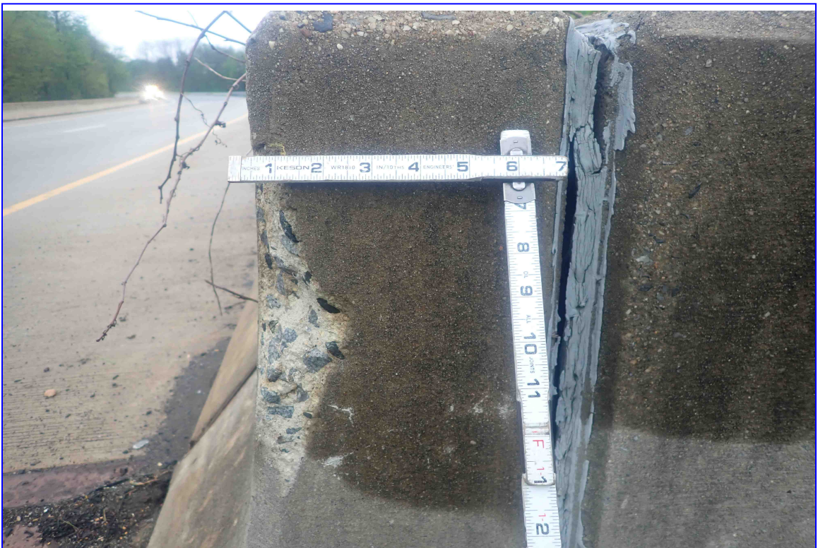
14. SPAN 1 SOUTH CONCRETE RAIL LARGE DEEP SPALL ON NORTHWEST CORNER LOOK E
