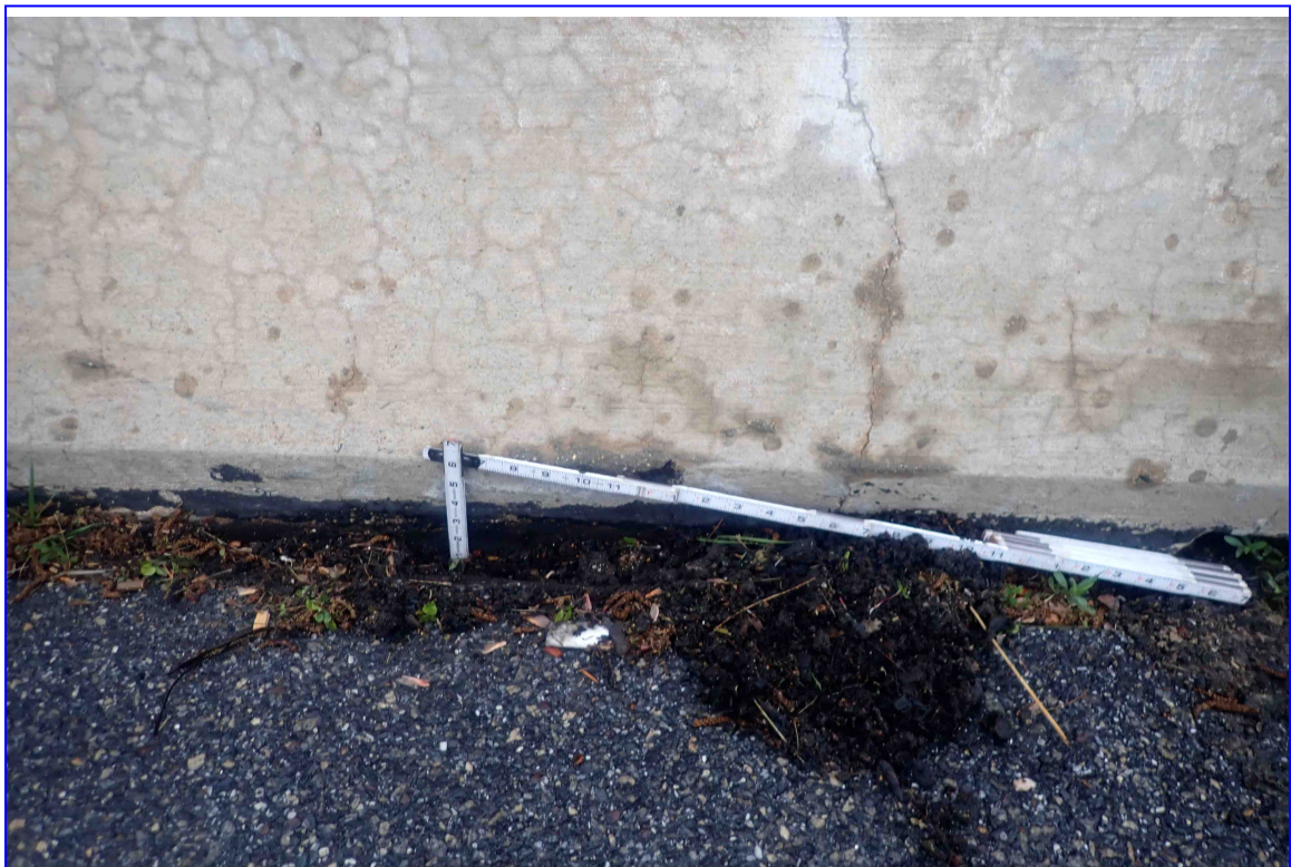
12. SPAN 3 POURED JOINT MISSING AT NORTHEAST WINGWALL PARAPET LOOKING N
