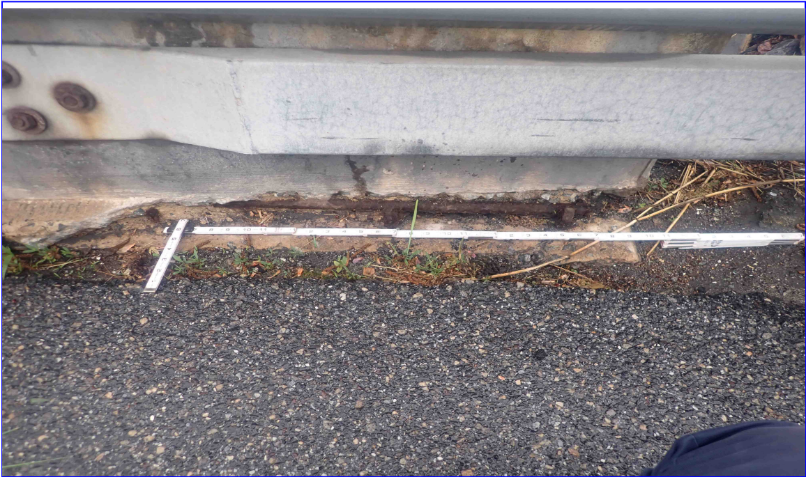
7. SPAN 3, NORTH CONCRETE RAIL EXPOSED PITTED BAR EAST END ON S FACE LOOK N
