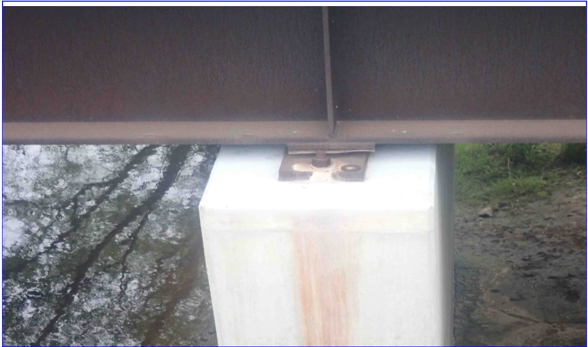
23. SPAN 3 E PIER 2 MOVE BEAR 1 SEPARATION TEPHLON PL & LG CORROS FLAKES LOOK E
