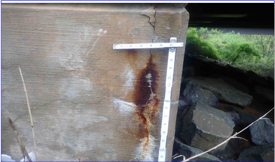
21. SPAN 3 EAST ABUTMENT BREASTWALL CRACK & RUST STAIN AT NORTH END LOOK S
