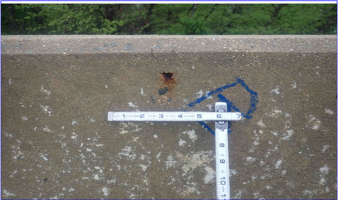
13. SPAN 2 NORTH CONCRETE RAIL SPALL & EXPOSED BAR ON SOUTH FACE LOOK N
