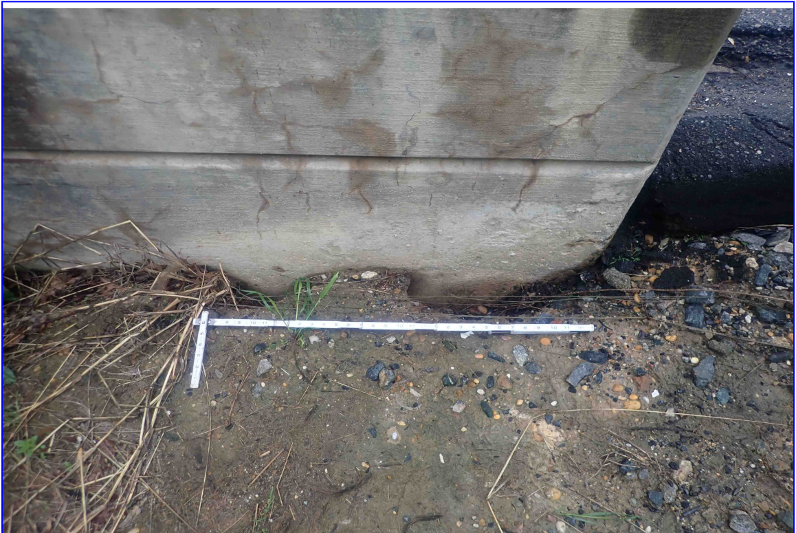
16. SPAN 1 EROSION HOLES AT NW NORTHWEST WINGWALL LOOKING SOUTH
