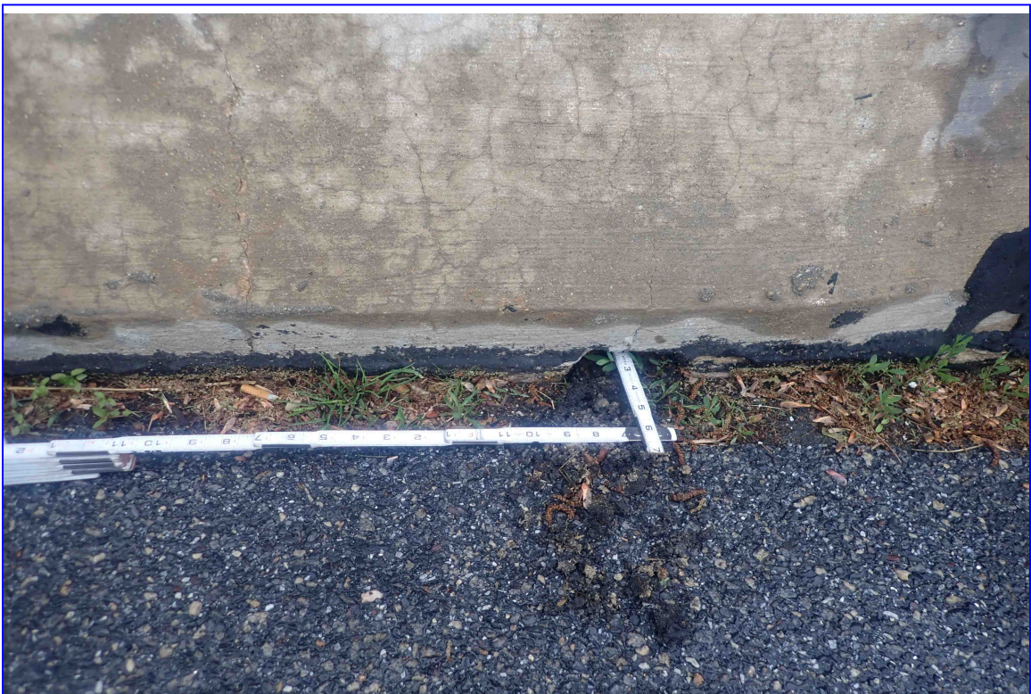
8. SPAN 3 NORTH CONCRETE RAIL, DEEP SPALL IN SOUTH CURB FACE LOOKING N
