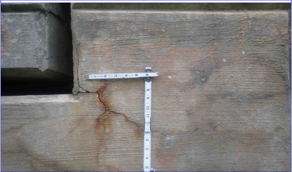
17. SPAN 1 W ABUT BACKWALL CRACK & RUST STAIN AT NORTH END ON N FACE LOOK S
