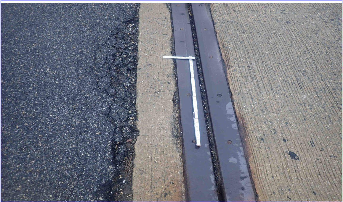
15. SPAN 1 STRIP SEAL JT HEADER LARGE SPALL RIGHT LN & APPR SLAB ASPH SPALL LOOK N
