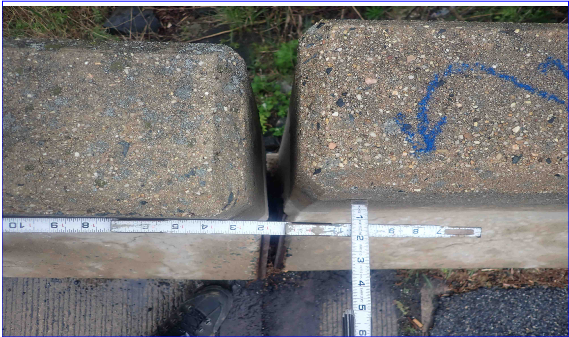
11. SPAN 3 NE WING/ RC RAIL SETTLED-TOP ROTATING N ~1-1/4" AT E ABUT LOOK N
