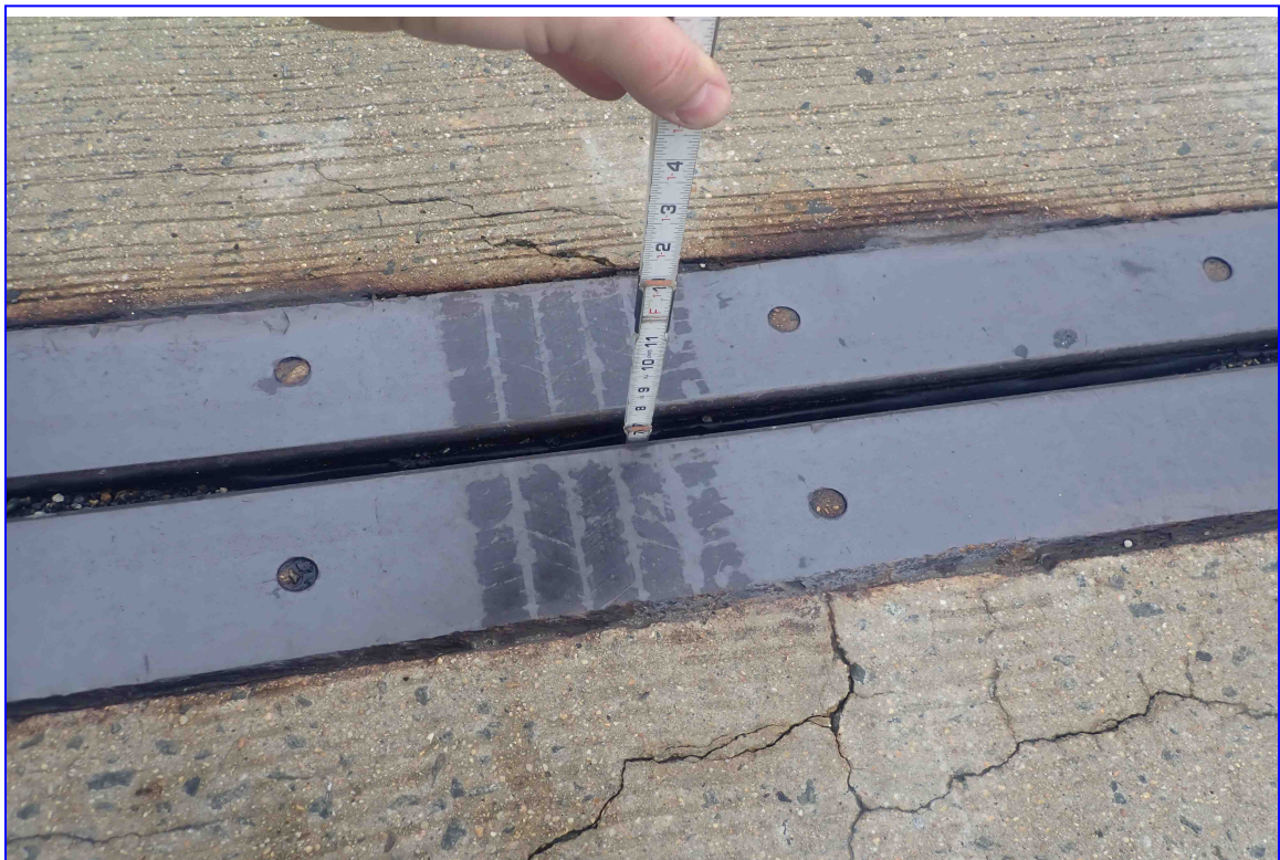
20. SPAN 1 STRIP SEAL GLAND IS TORN IN LEFT LANE NEAR WHITE LINE LOOK DOWN
