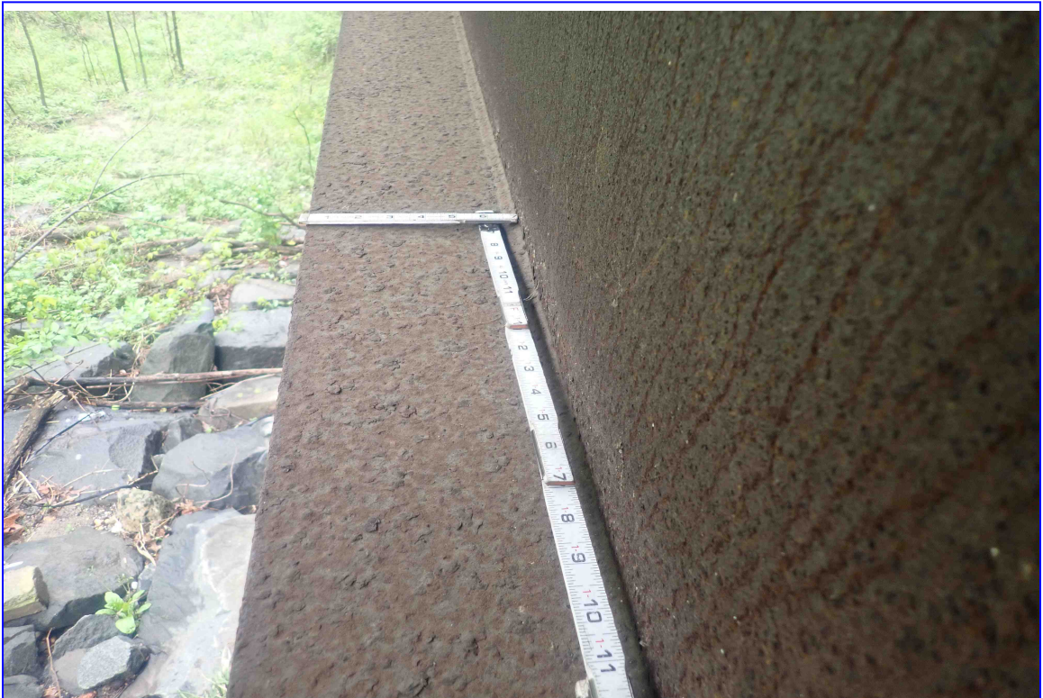
18. SPAN 1 N FACIA GRDR 1 HAS ~1/4 INCH CORROSION FLAKES ON TOP OF BOT FL LOOK E
